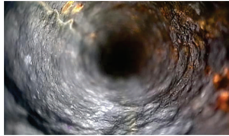
Real-Life Problem 2 Corrosion of Piping
